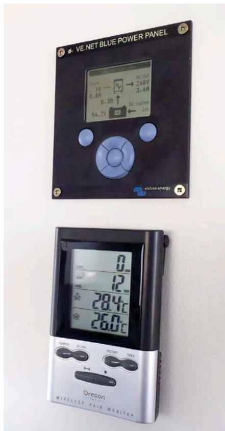
↑ The remote panel for the Victron inverter (top) and the Oregon rain monitor let Vadim keep an eye on things.
