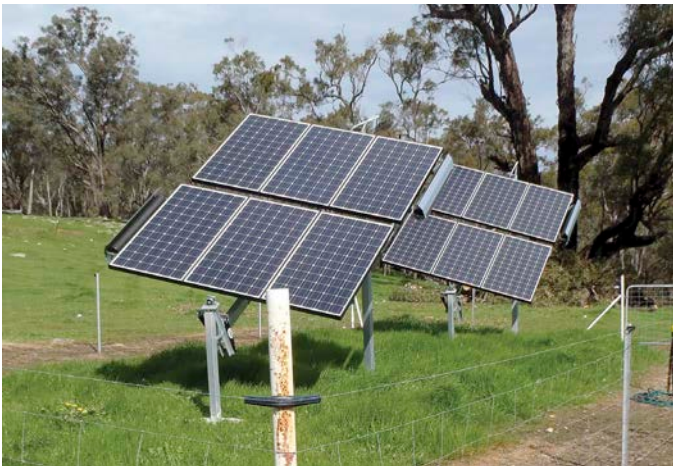
↑ The 12 solar panels on their trackers provide most of the Shouse's energy needs during summer.
