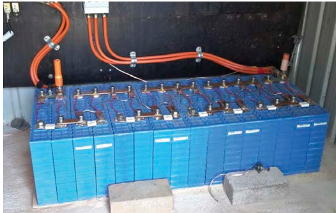
← Gordon's battery bank is rated at around 21kWh. On some days he uses more energy than the bank's capacity due to the high input from the charging sources. Note that it would normally have a cover over the terminals for safety.
